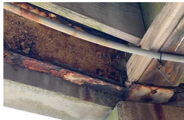
2.3b Deteriorated Ledgers and Beam Seats Supporting Wood Deck Framing
