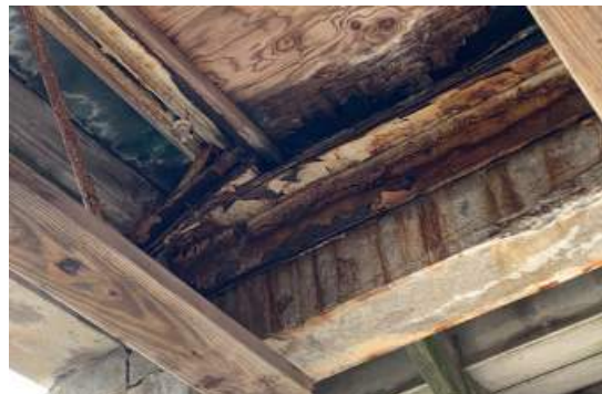
1.2b Severe Joist Deterioration
