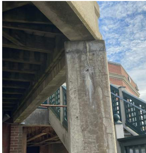
39. Cracking on concrete structure at second floor framing.
