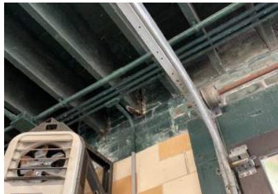
3.1a Localized End Deterioration of Wood Joists/Beam
