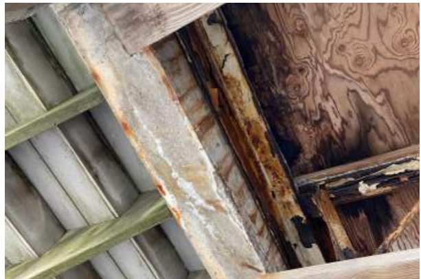
58. Spalling and exposed reinforcing steel on concrete beam.
