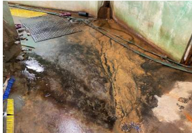
35. Water penetration at joint between Carousel building and Rotunda building.
