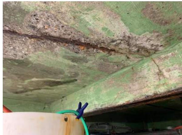
2.1a Deteriorated First Floor Slab and Beams
