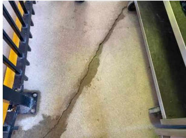
41. Cracks in second floor concrete slab.
