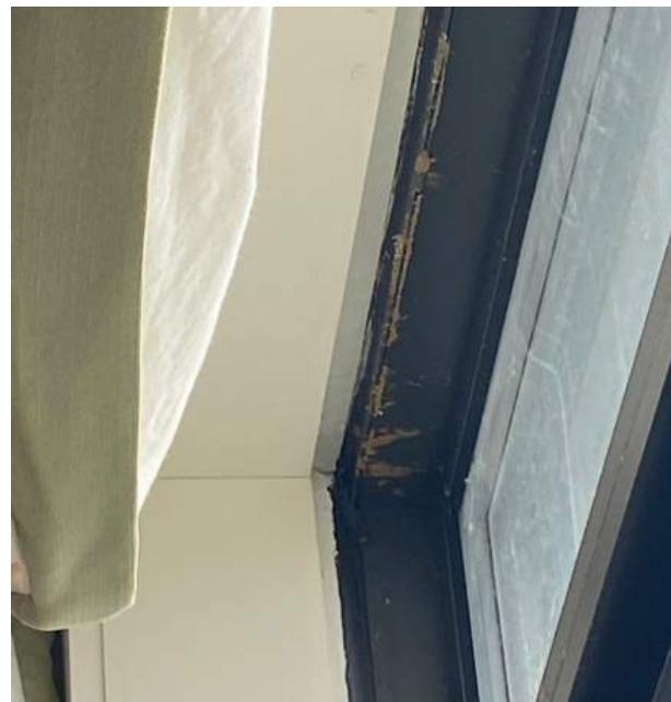
27. Result of water infiltration at window head.
