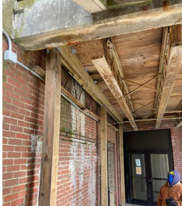
57. Extreme corrosion on painted steel bar joists.
