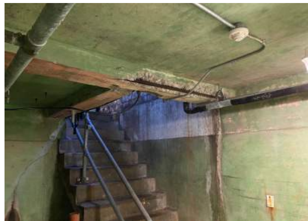
36. Concrete loss resulting in corrosion of reinforcing steel members.
