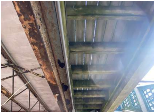
51. Heavy corrosion on steel framing.
