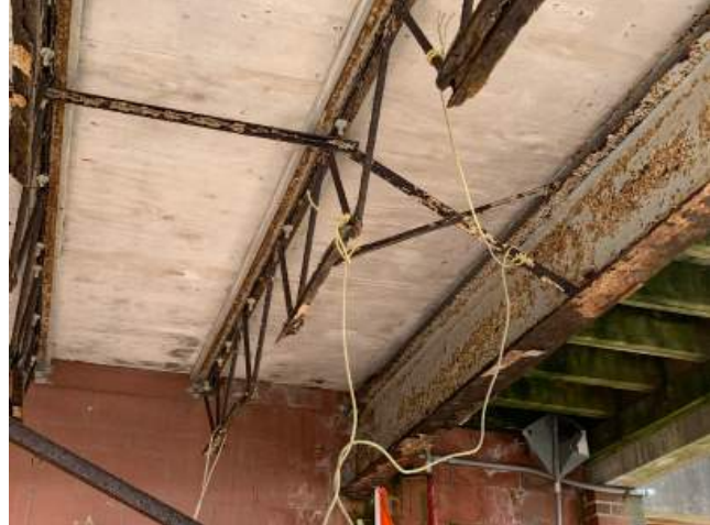
1.1a Severe Joist Deterioration
