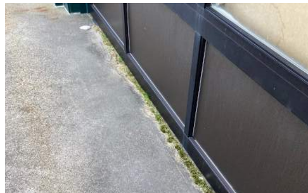
59. Moss growth indicating prolonged periods of moisture.
