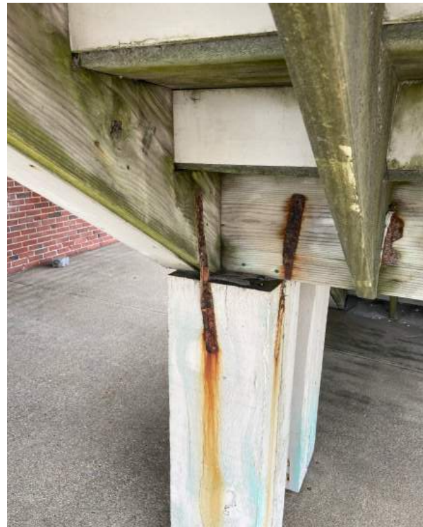
65. The strap anchors connecting the stair stringer to the wood post supports should be replaced due to corrosion.
