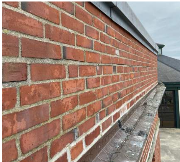
13. Masonry above cornice on second floor requires repointing .
