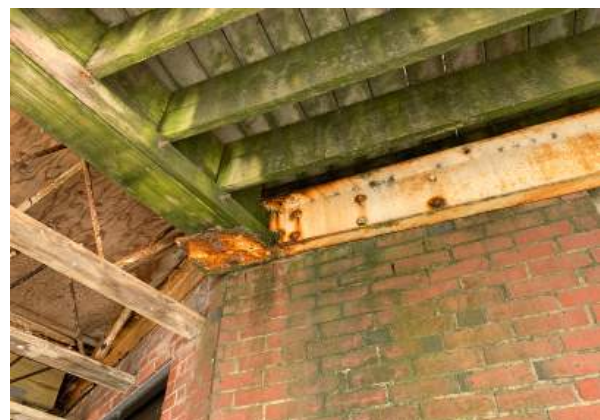
2.3a Deteriorated Ledgers and Beam Seats Supporting Wood Deck Framing
