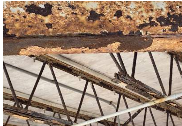
38. Corrosion on steel framing at second floor.
