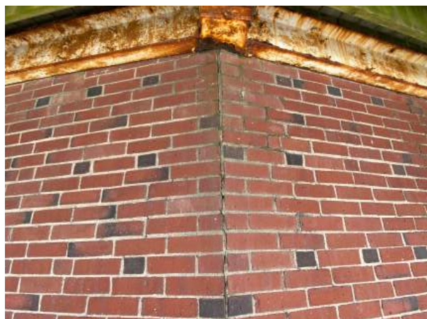
14. Joints cracking at the corner of the building.
