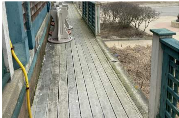
61. Section of missing railing
