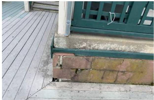
3.2b Deterioration of CMU Walls
