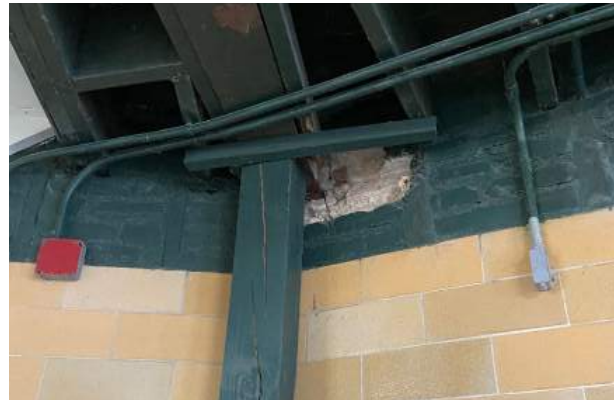
26. Photos of deteriorated wood joists at the intersection of the masonry wall.
