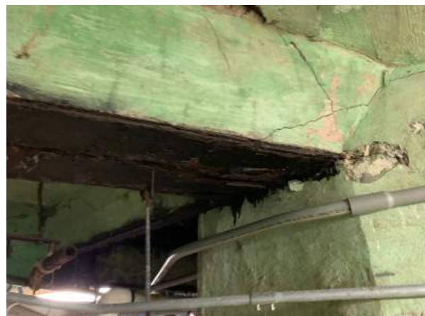
2.1b Deteriorated First Floor Slab and Beams
