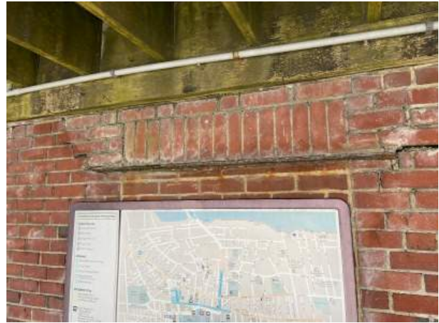
45. Cracking, failing masonry joints and biologic growth on south and west side at the first floor.
