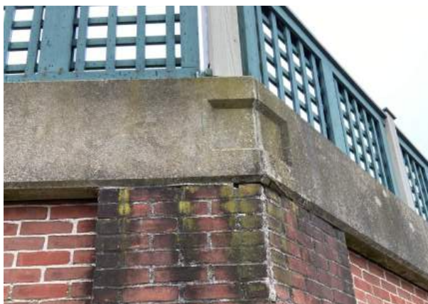
30. Black and green stains on masonry as a result of water drainage and biologic growth.
