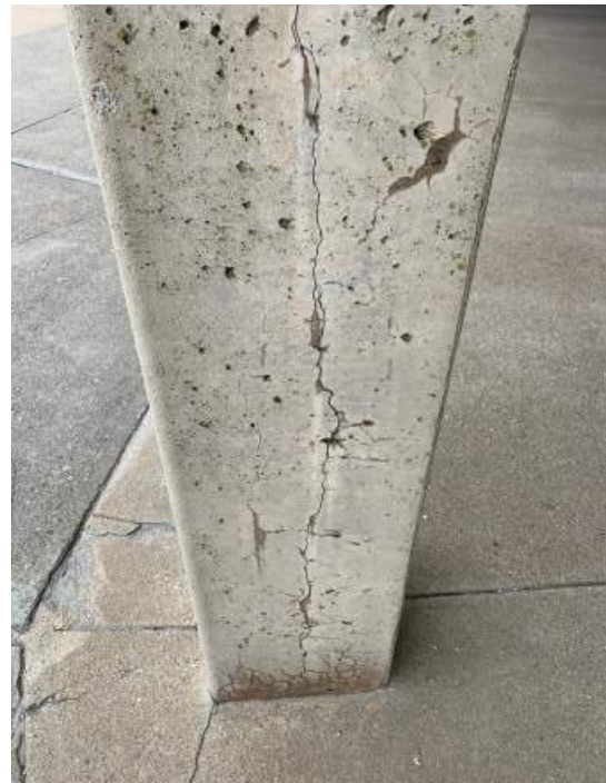
3.3b Cracks in Concrete Piers
