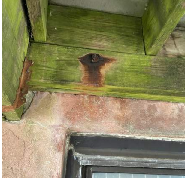
54. Rust colored water weeping through the ledger boards.
