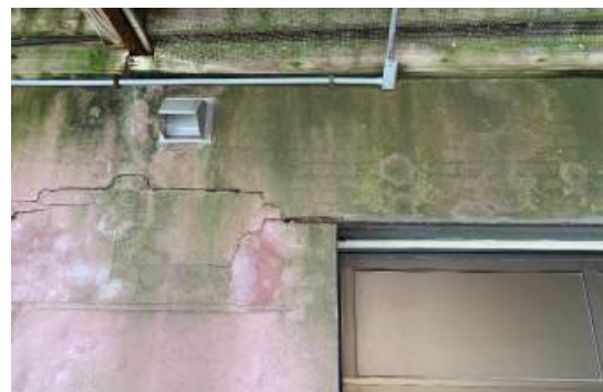
3.4b Rust Jacking of Steel Lintels
