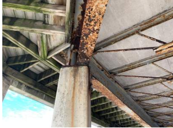
2.2a Deteriorated Column Bases and Beams
