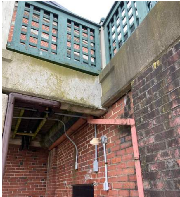
55. Structure has settled along outer edge of boardwalk.
