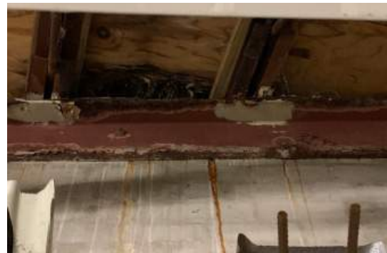
2.4b Localized Joist and Joist Seat Deterioration
