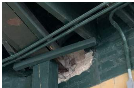
3.1b Localized End Deterioration of Wood Joists/Beam
