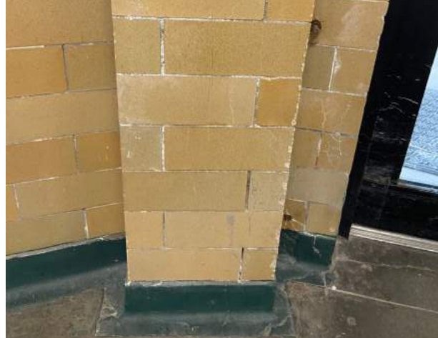
24. Cracked areas on blocking.
