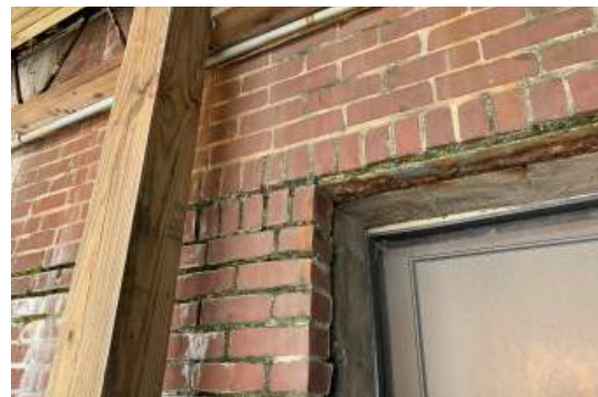
3.4a Rust Jacking of Steel Lintels
