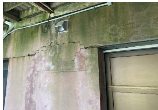
44. Rust, cracking and biologic growth on north wall at the first floor.
