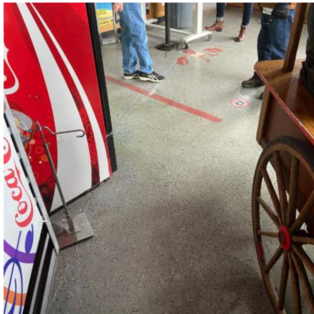
50. Crack in the concrete slab.
