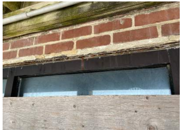
46. Rust jacking of steel lintels over doors and windows.
