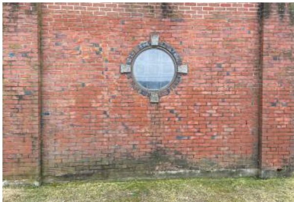
31. Black stains on masonry as a result of water drainage.
