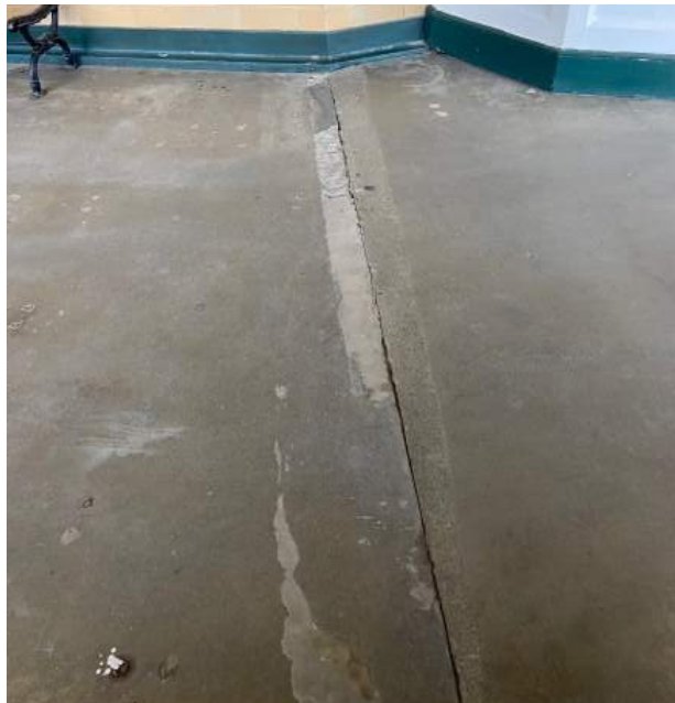
25. Cracking in slab-on-grade at first floor level.
