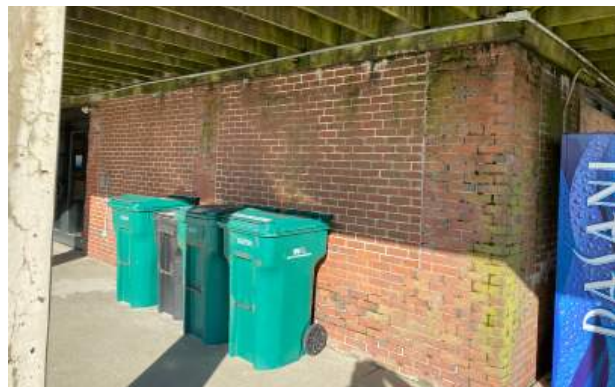
47. Masonry joints need repointing
