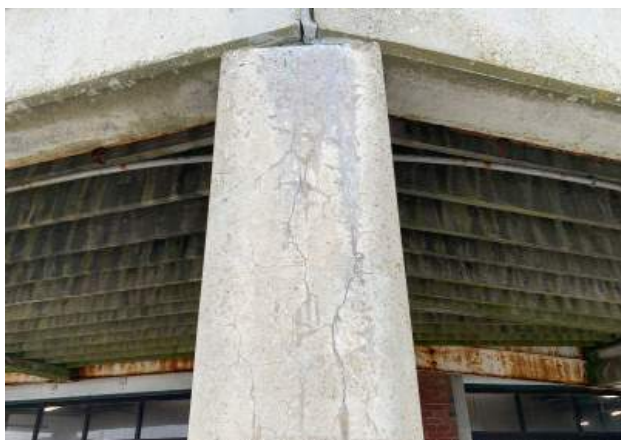
3.3a Cracks in Concrete Piers
