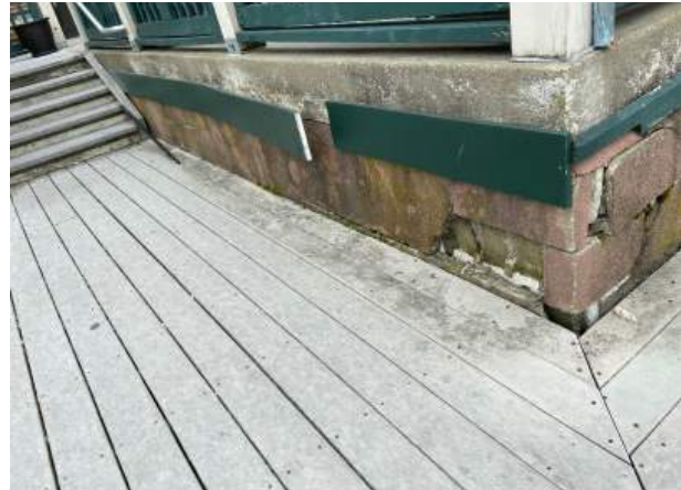
48. PVC trim board breaking apart.
