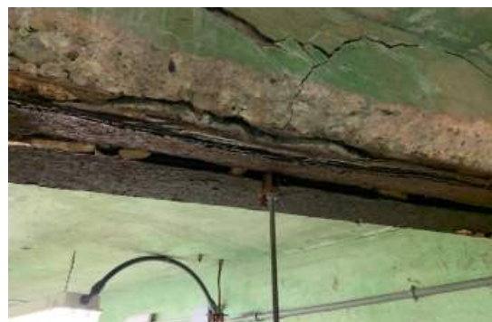
1.3b Deteriorated First Floor Slab and Beams
