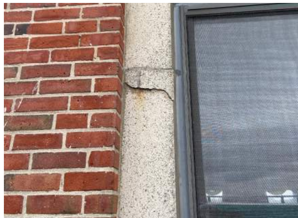
20. Spalling at window area.
