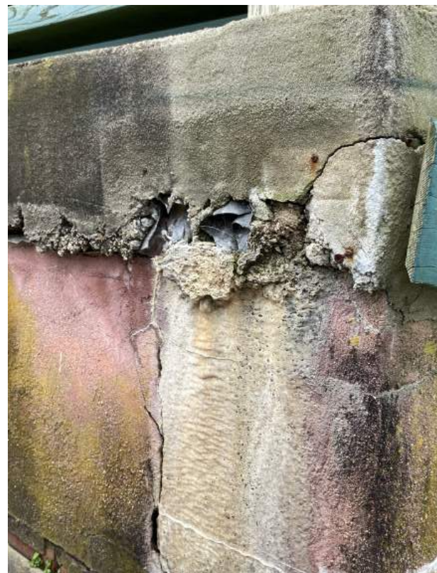
49. Wall damage and spalling from water infiltration
