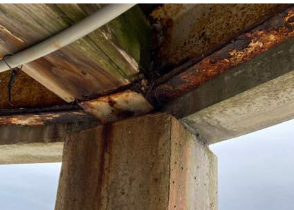
53. Corrosion on steel channel ledgers and steel saddles.
