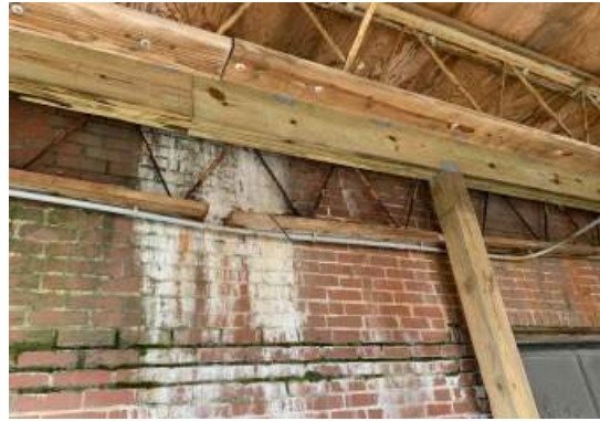
1.2a Severe Joist Deterioration
