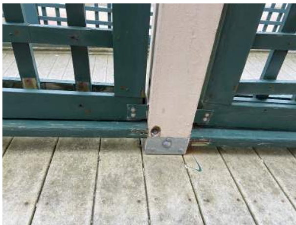
63. Loose connection where flange connects to wood post.
