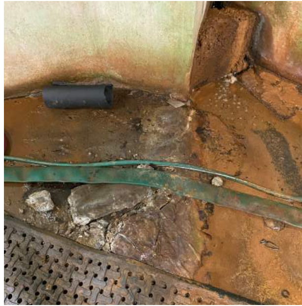
21. Water infiltration in basement
