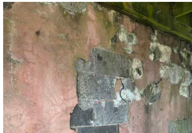
43. Spalling, biologic growth and deterioration on first floor exterior wall.
