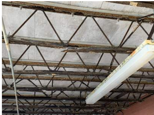
1.1b Severe Joist Deterioration
