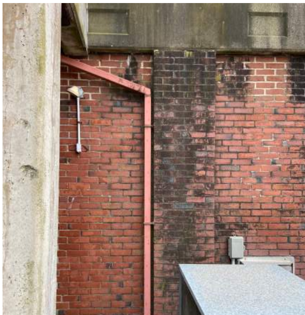
29. Black stains on masonry as a result of water drainage.
