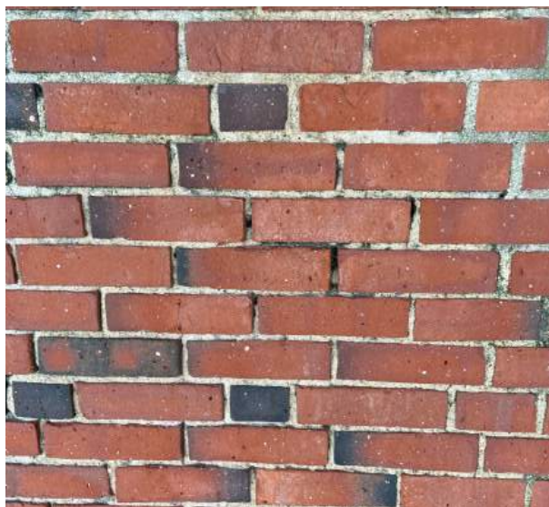
15. Areas on south facing elevations require repointing.
