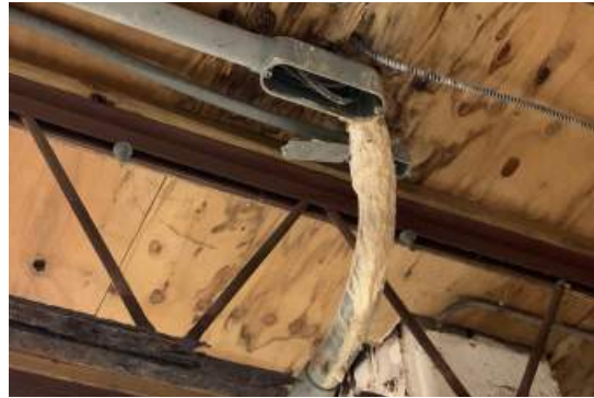
2.4a Localized Joist and Joist Seat Deterioration
