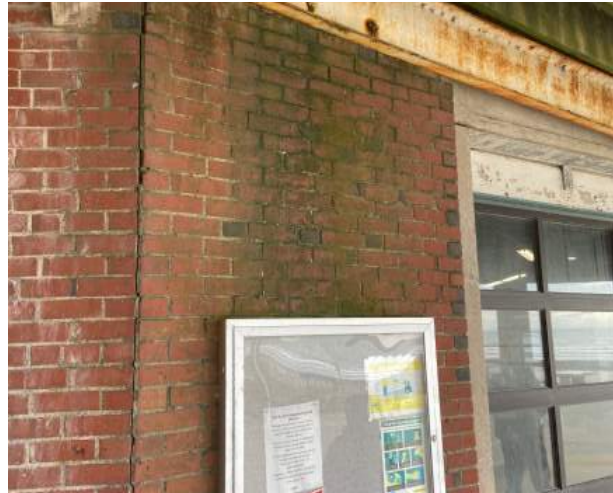
16. Heavy biologic growth on brick masonry walls.
