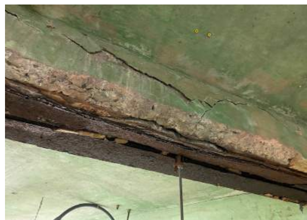
37. Corrosion on underside of beam.
