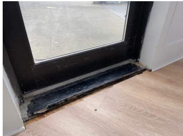
25. Potential trip hazard.
