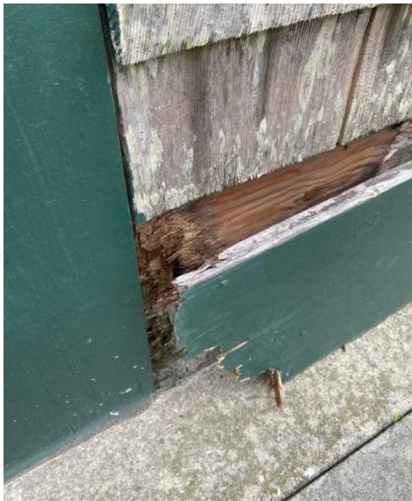
32. Deteriorated trim and sheathing behind it.
