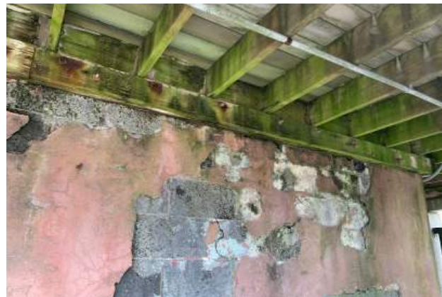
3.2a Deterioration of CMU Walls
