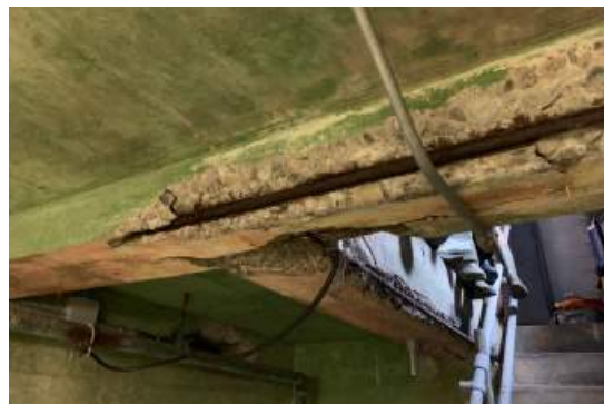
1.3a Deteriorated First Floor Slab and Beams
