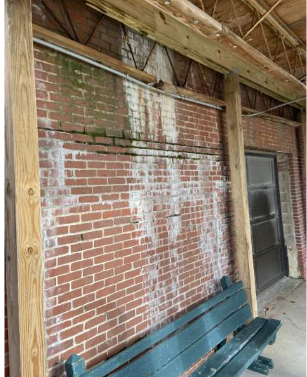
33. Efflorescence on brick masonry near overhead door.
