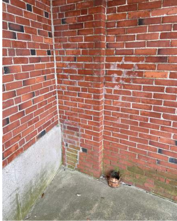
66. Broken pipe with jagged edges presents safety concern.
