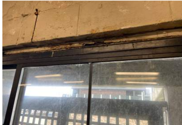
49. Signs of water infiltration on east wall window.
