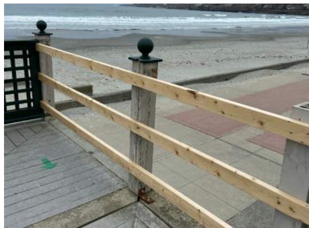
62. Section of missing railing.
